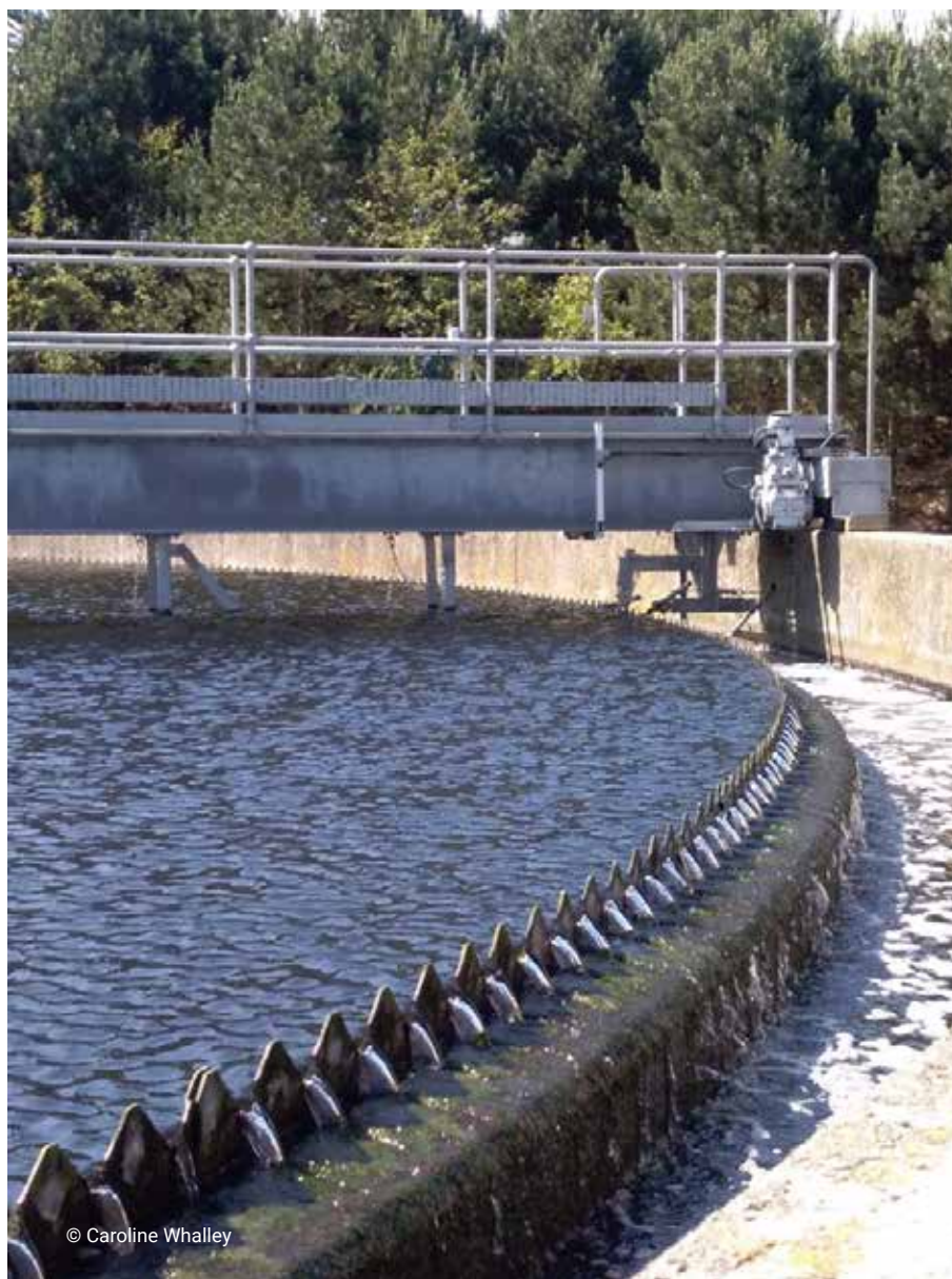
Figure 3.4 Aeration in urban waste water treatment
